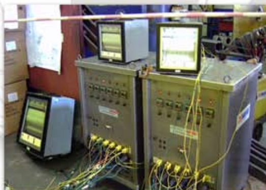
50 AMP KVA's with build in programmers
